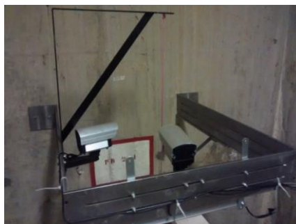
Fig. 5. Automated reading system installed in direct pendulum.
