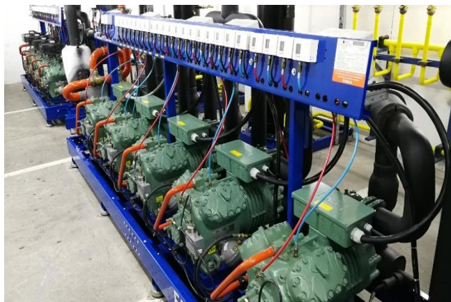
Fig. 1. R404A refrigeration system.
